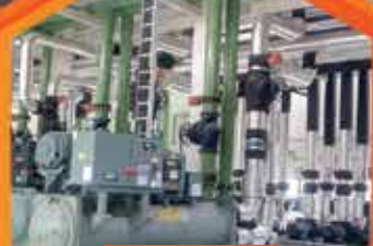
Air Conditioning and Ventilation
